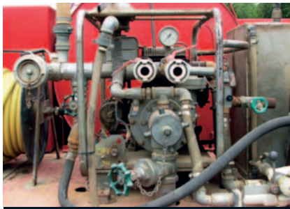
Original pump with non original hose reels, class A foam system and lockers
